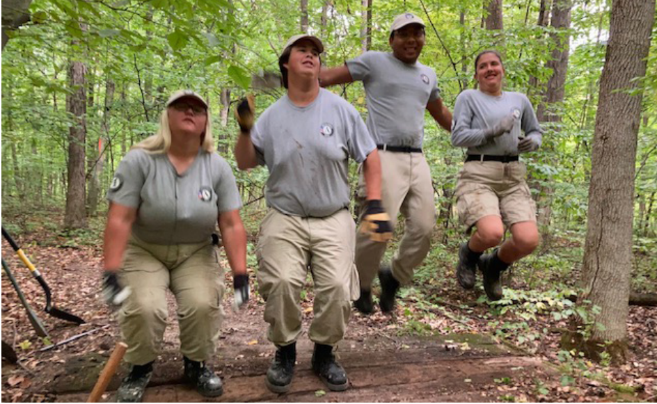
Americorps workers jump on new railroad ties to seat them into their bridge.
